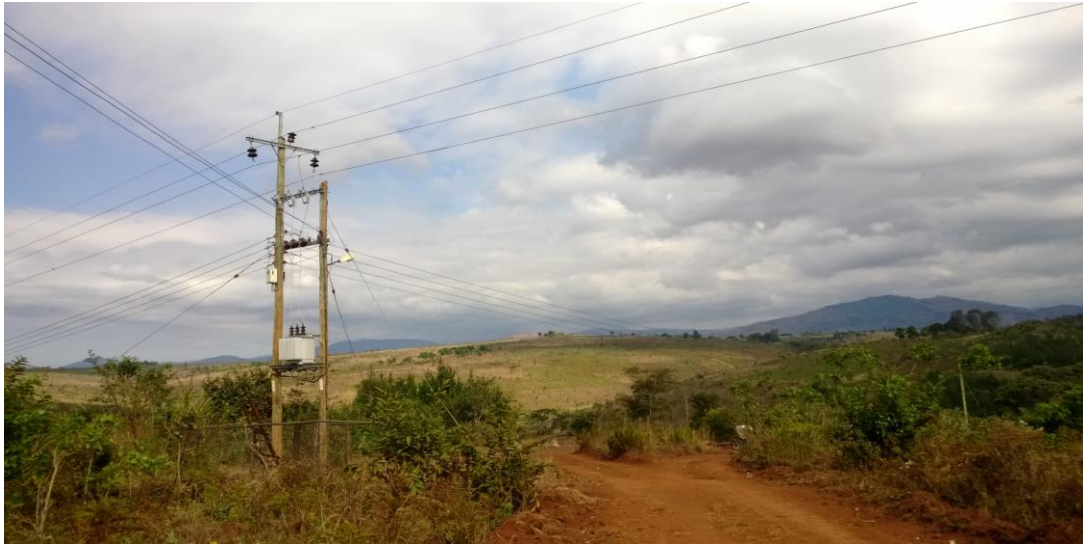
Figure 4: View of the mini-grid network at Mbanga, Ruvuma Tanzania
