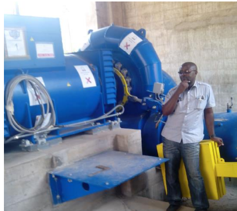
Figure 2: View of the 500 kW turbine installed at Andoya power plant
