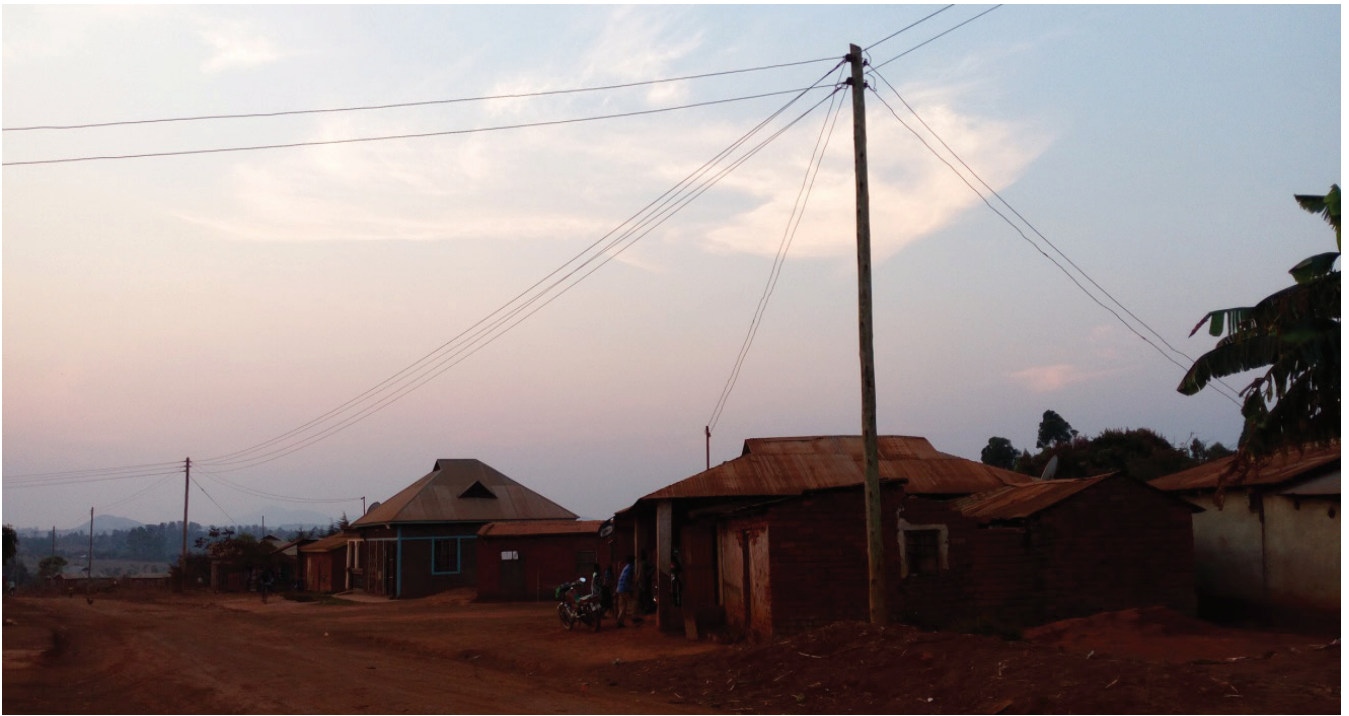
Power distribution line for Andoya mini hydropower , Kifakara village, Mbinga District
