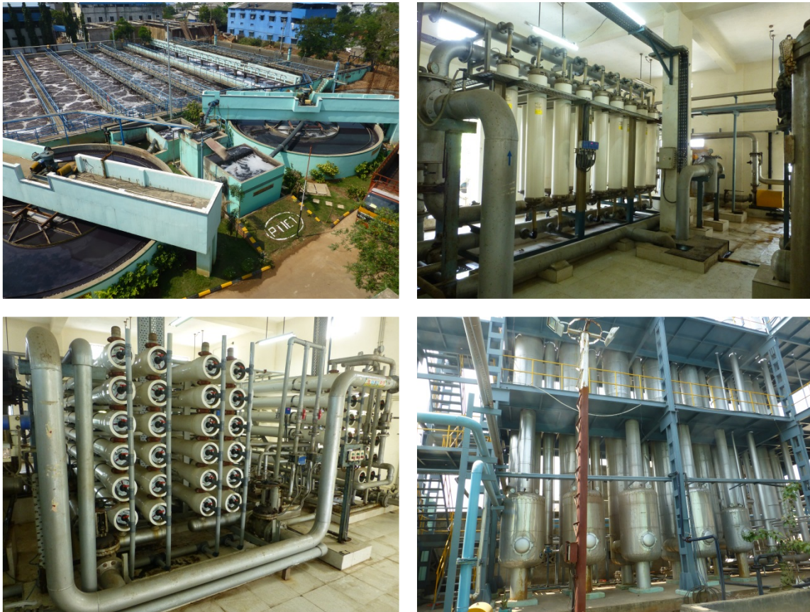
Figure 3. Pallavaram CETP, Aeration and clarifier tanks; Ultrafiltration units; Reverse osmosis; Multiple evaporators
