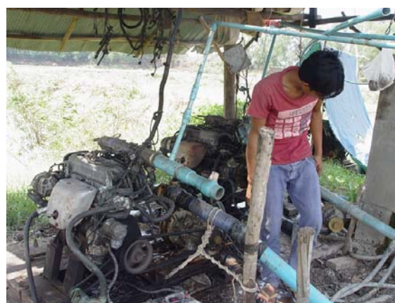
Figure 76: Biogas fuelled water pumps
