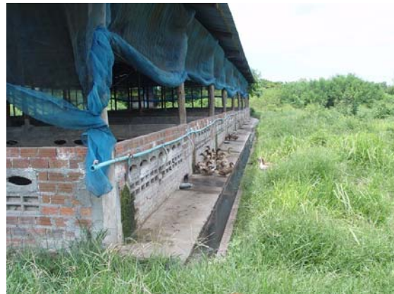
Figure 26: Facility for waste water removal
