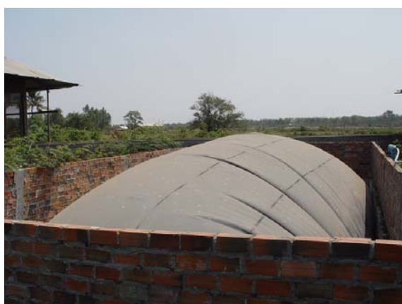
Figure 75: 250 m 3 biogas system at Taing Haing Ly
