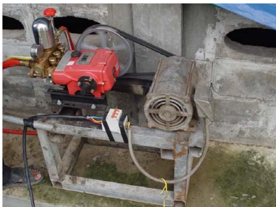
Figure 51: Pump for water pressurisation
