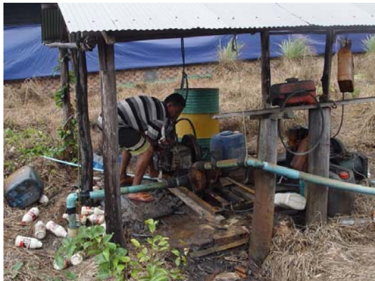
Figure 35: Water pump at Te Sopheak farm
