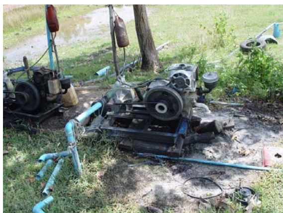
Figure 27: Diesel fuelled water pump
