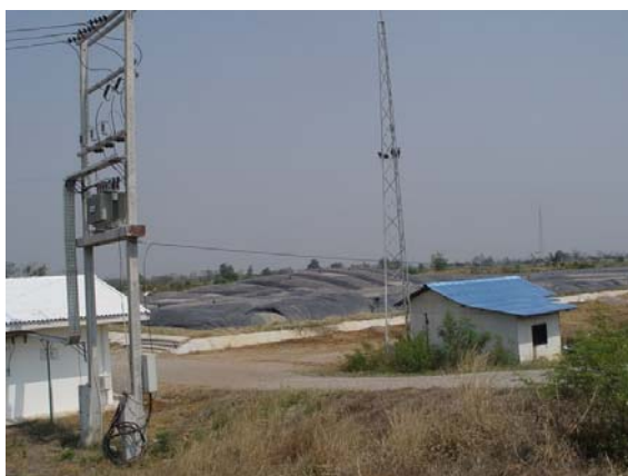
Figure 9: BAI biogas plant
