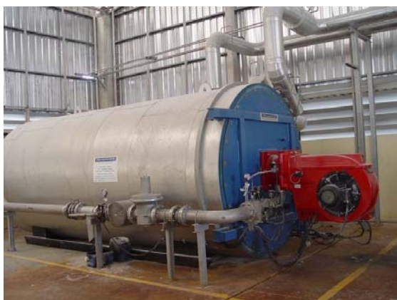
Figure 11: BAI thermal oil heater
