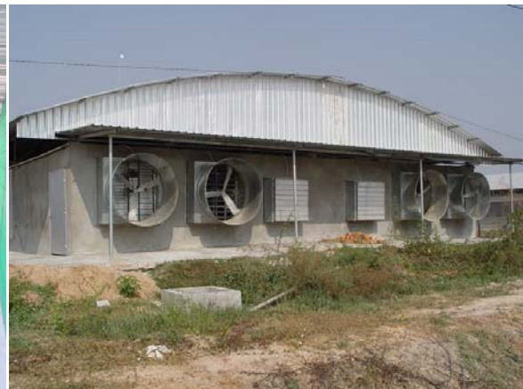
Figure 4: Draught fans in the back of closed stable
