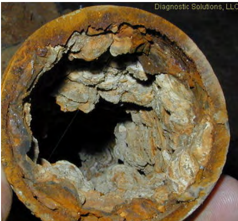
Fig. 4.2. Water distribution pipe with significant tuberculation (courtesy of Diagnostic Solutions)
