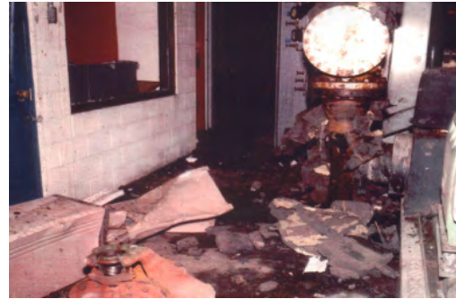
Fig. 6.2. Explosion due to closed valves on both sides of a pump
