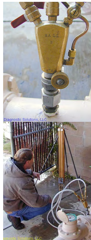
Fig. 12.21. Flow Reading with a Multi-port Pitot Tube
