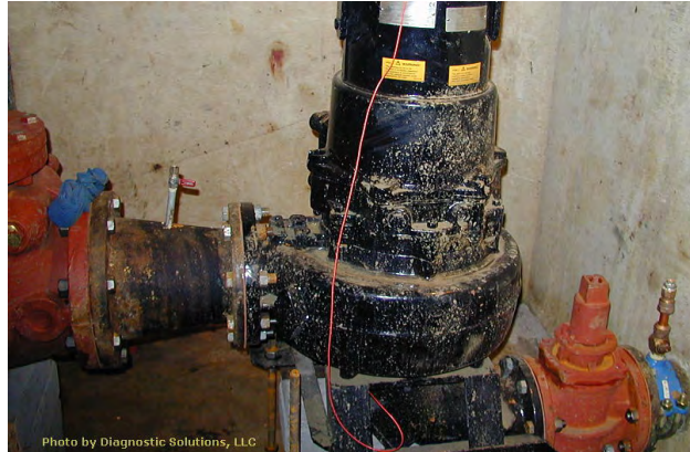
Fig. 12.16. Taps for Measuring Suction and Discharge Pressure
