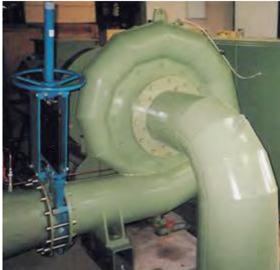
Fig 22: Horizontal Francis Turbine
