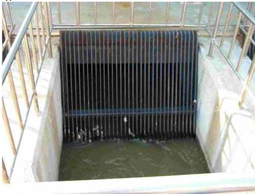
Figure 1. Typical bar screen
