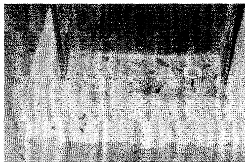
Residue by silos column in main mill areas
