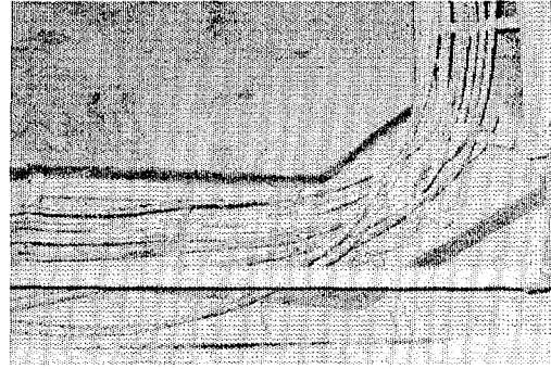
Cable tray spillage
