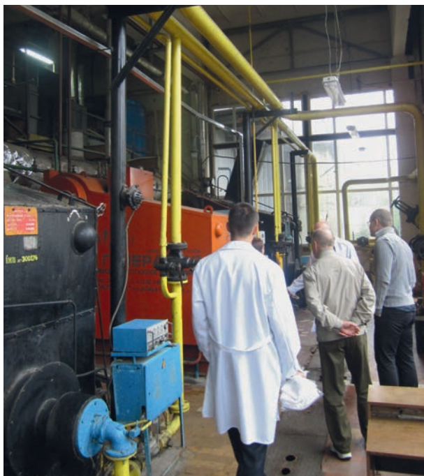
Installation of heat exchangers at one of the leading industrial bakeries in Ukraine.
