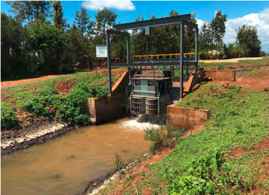
Ultra-low heat micro hydropower installation in Mwea, Kenya
