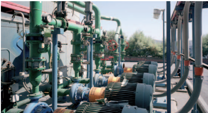
Industrial motor-driven pumps system
