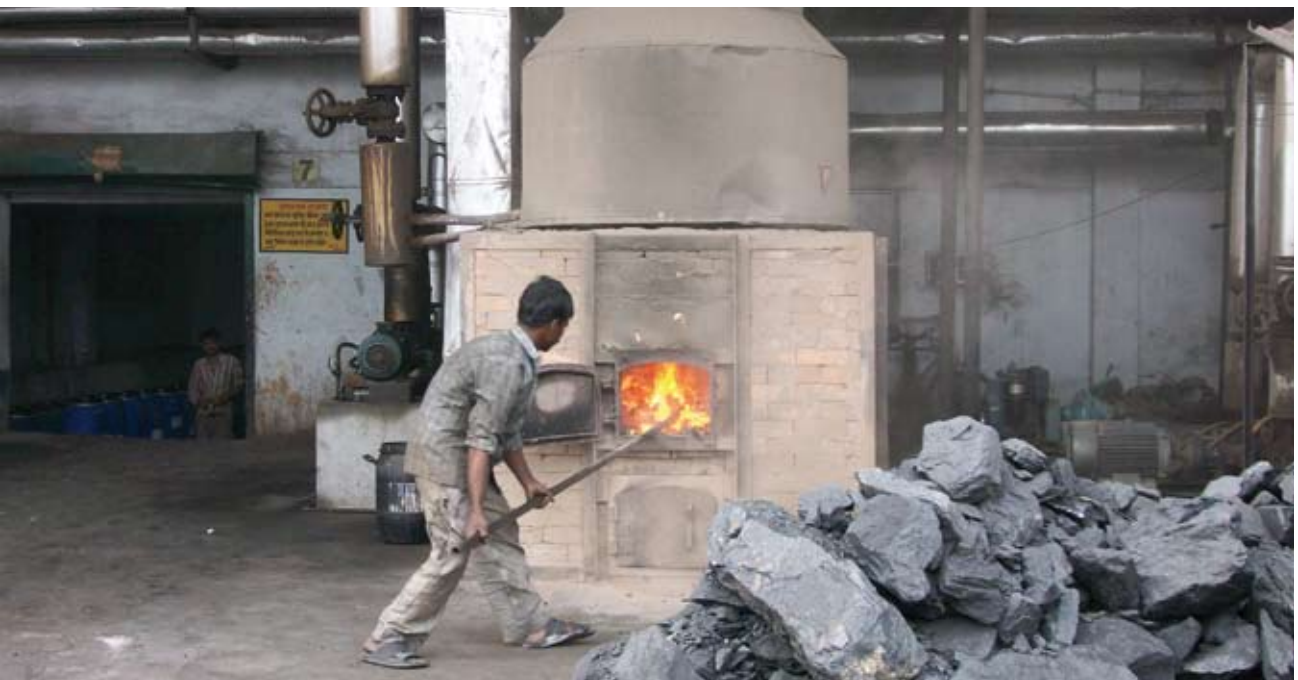
Coal boiler in India
