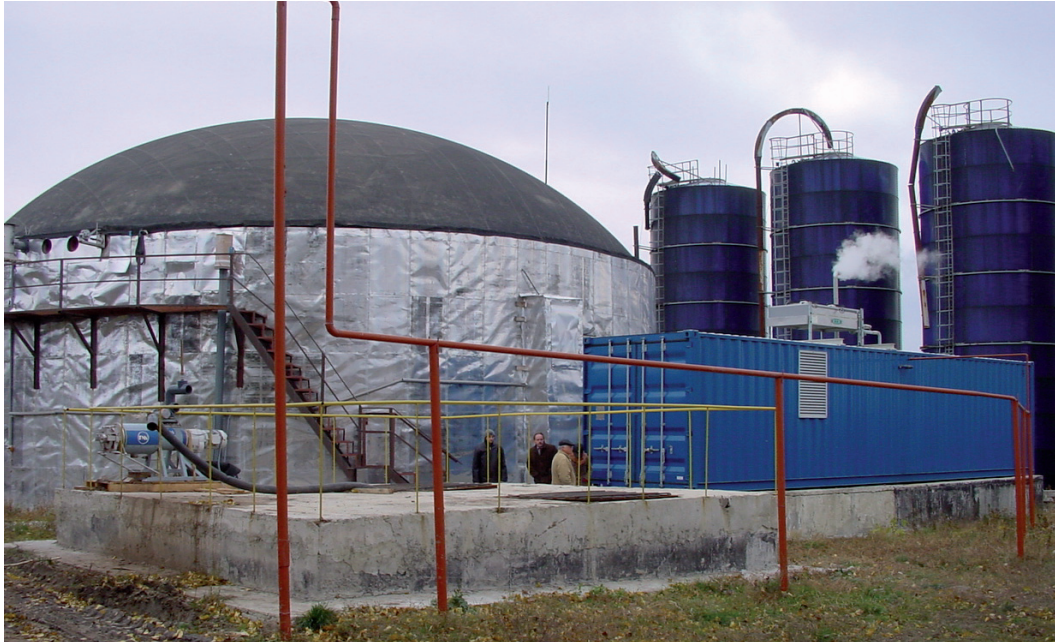
Figure III. Cow manure digester in Moldova
