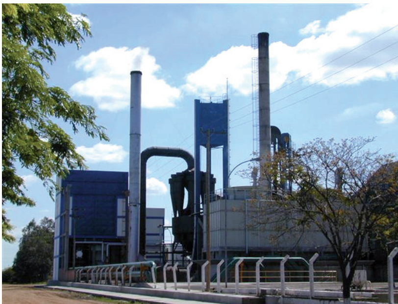
Figure XVII. The CHP plant at CAMIL Itaquí [63]
