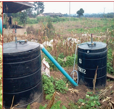
Installed biodiesel facility
