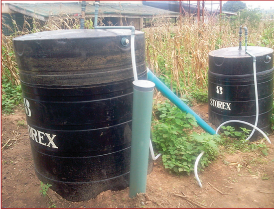
Biodiesel facility connected to the factory
