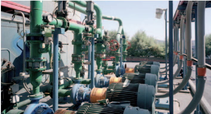
Industrial motor-driven pumps system
