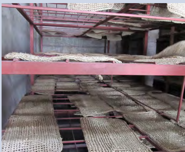
FIGURE 8. A woman using seagrass drying equipment (top), and a drying chamber, both provided by UNIDO
