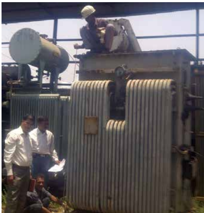
Figure 6: PCBs collection from transformers
