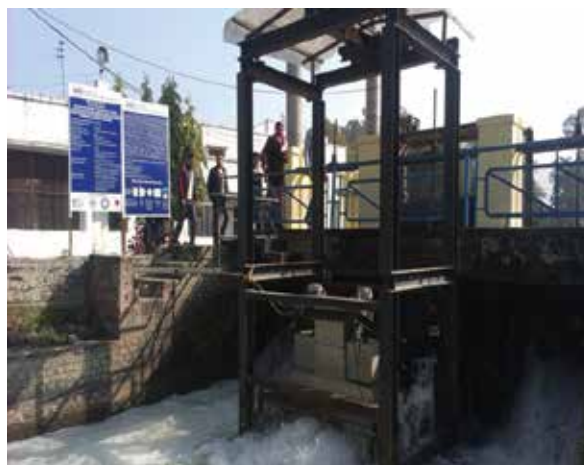
Figure 10: Ultra low-head micro hydro plant in Uttarakhand
