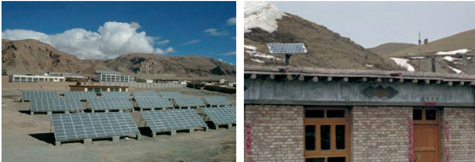
Figure VII. Examples of SDDX installations in China
