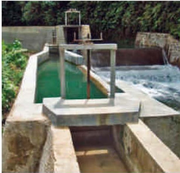
Intake of small hydropower plant in Indonesia.
