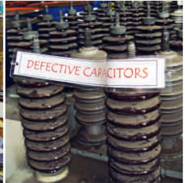
Philippines: stockpiles of capacitors for disposal.
