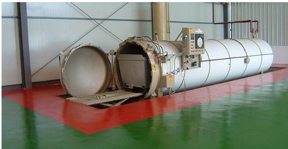
UNIDO helps upgrade medical waste disposal equipment in China
