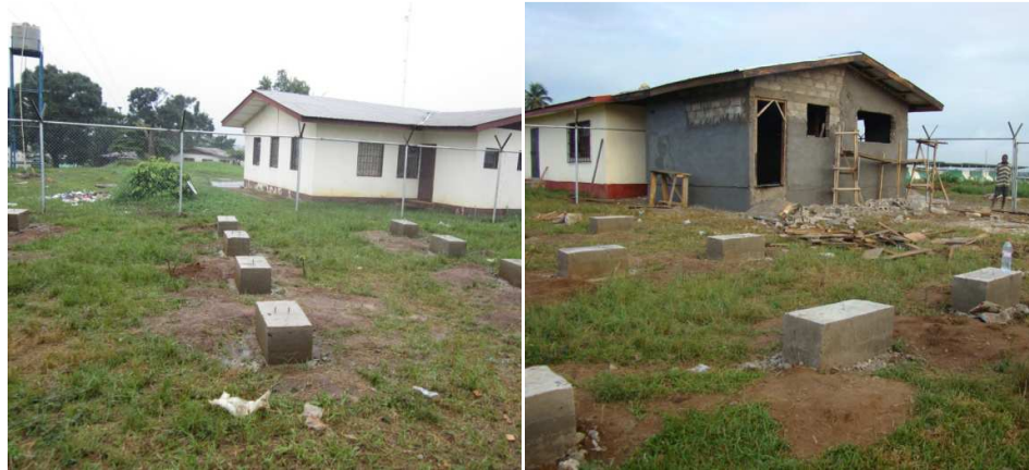
Figure 15 - Ganta 15 kW PV system in construction (MYS building on left and battery house on right)
