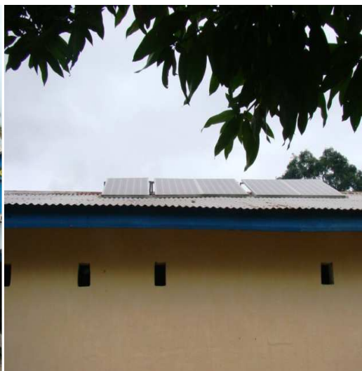
Figure 3: Existing 1 kW PV system in Pujehun
