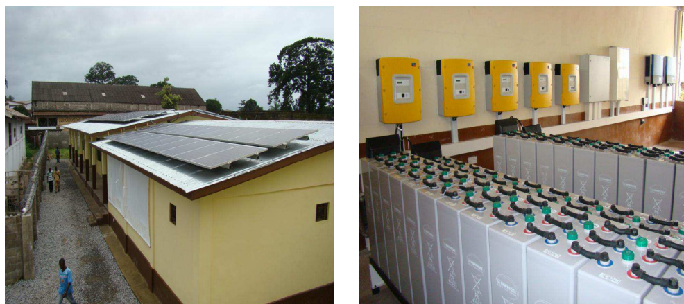
Figure 16 - Bo Growth Centre 25 kW PV system fully installed
