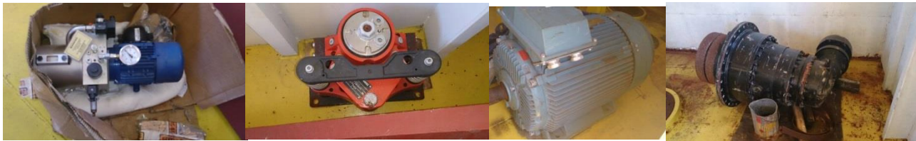
Pictureset 2: Hydraulic pump, hydraulic break, generator, gears (stored inside platform)
