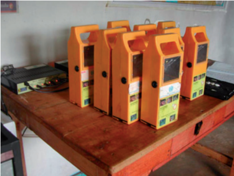
Kirinyaga (Kenya): Battery charging
