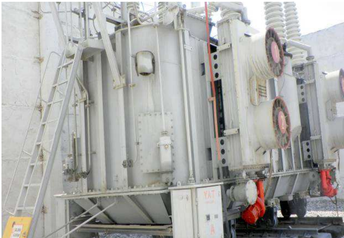
Picture 3. Transformer of 125 megawatt at Azerenergy. Installed in 1993. Content 47 tons of oil without PCB.
