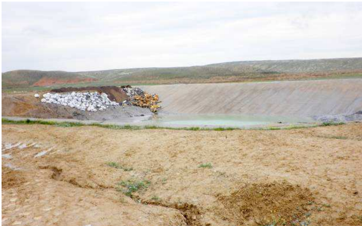
Picture 8. The new Landfill of the National Center for Waste Management in Abscheron region
