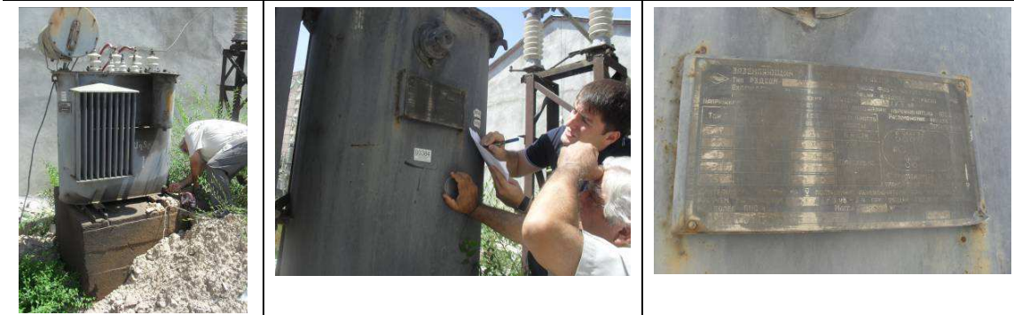
Facility: Shaumyan-1 110 kV substation “Electric Network of Armenia”
