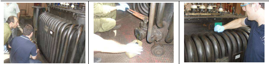
Facility: Yerevan-1 HPP “The International Energy Corporation”
