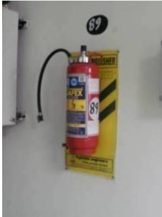
Figure 31: Typical powder type fire extinguisher
