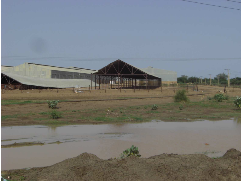
Figure S5 One of the sheds has collapsed
