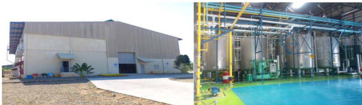
Fig. 2.5.2-1. The Non-Combustion PCB destruction facility in Mariveles, Bataan
