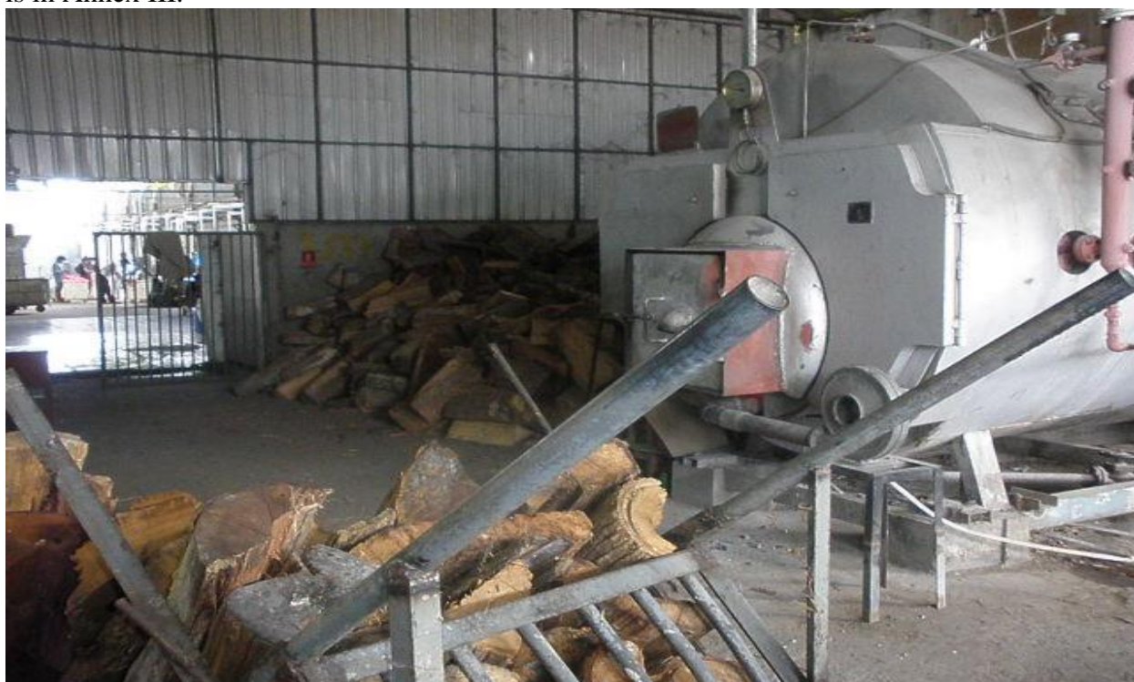
Cambodia: A boiler heating with wood in one of the demonstration companies.
