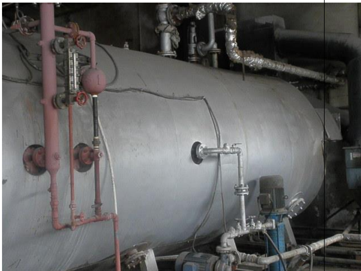
Cambodia: An industrial boiler
