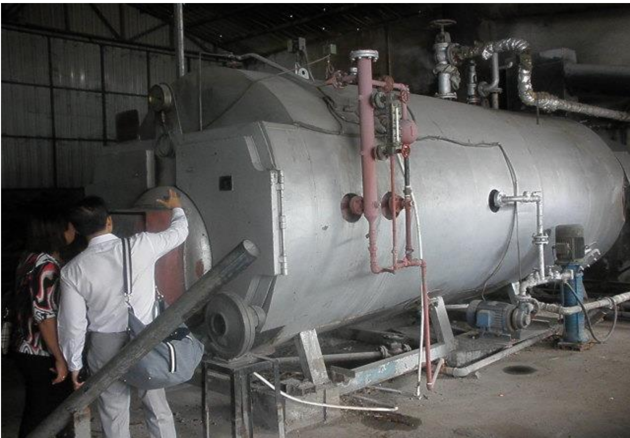
A boiler in one of the demonstration pilot enterprises.
