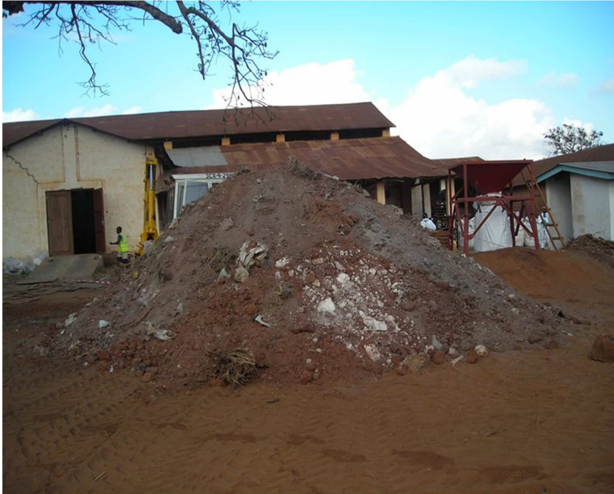
NHC site in Morogoro during the excavation of soil a few years ago
