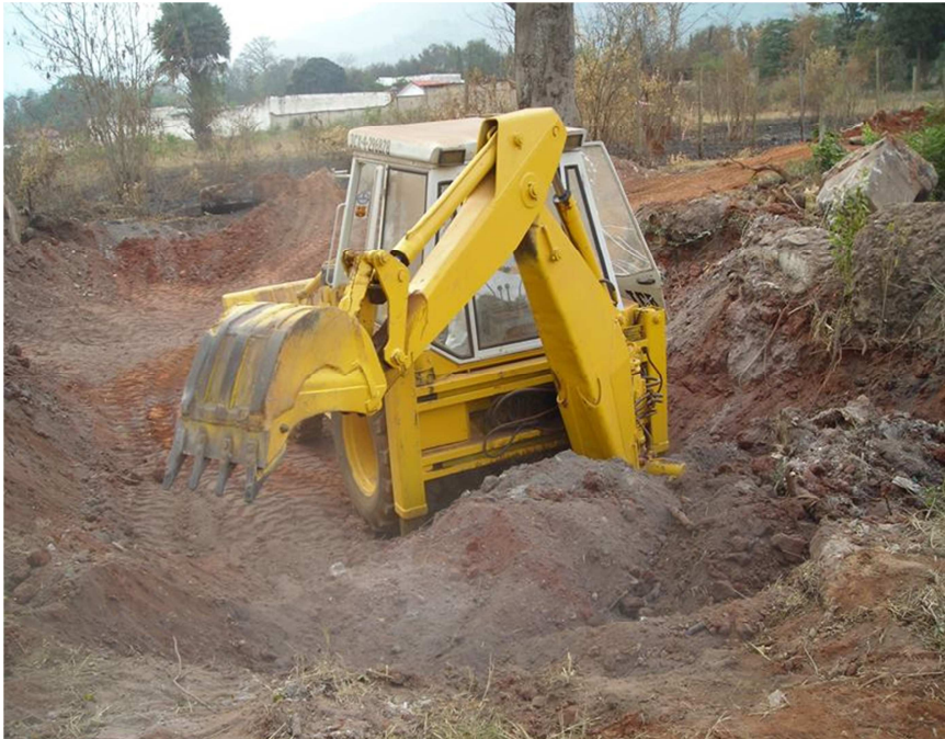
NHC site in Morogoro during the excavation of soil a few years ago
