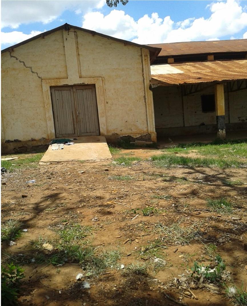
The main building of the abandoned NHC site in Morogoro- Dec. 11 th , 2013
