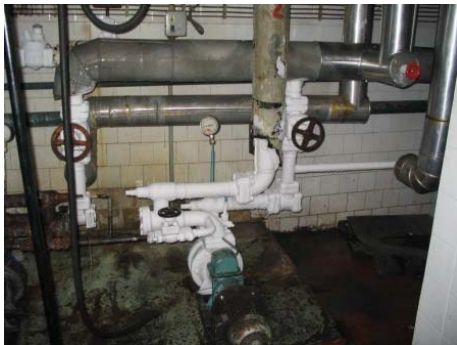
Cooling plant, missing insulation on the pipeline and valves
