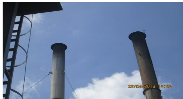
Emissions after RECP Implementation
