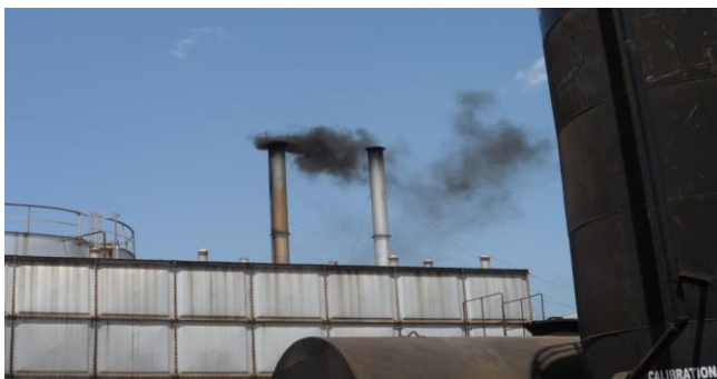
Emissions from the Boiler Before RECP
