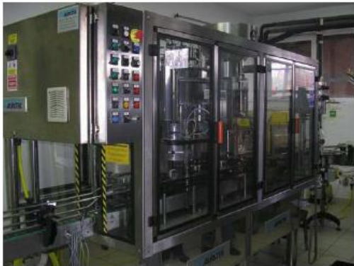
Packing and labeling equipment
