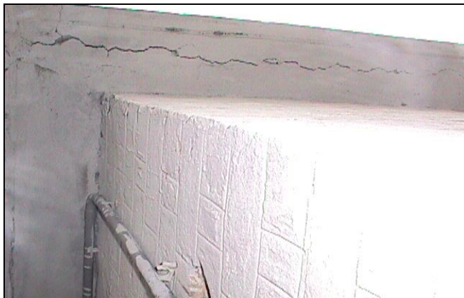
Before Installation Experimental Roof showing cracks
