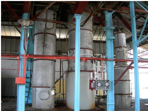
Figure 1. Insulated distillation columns
