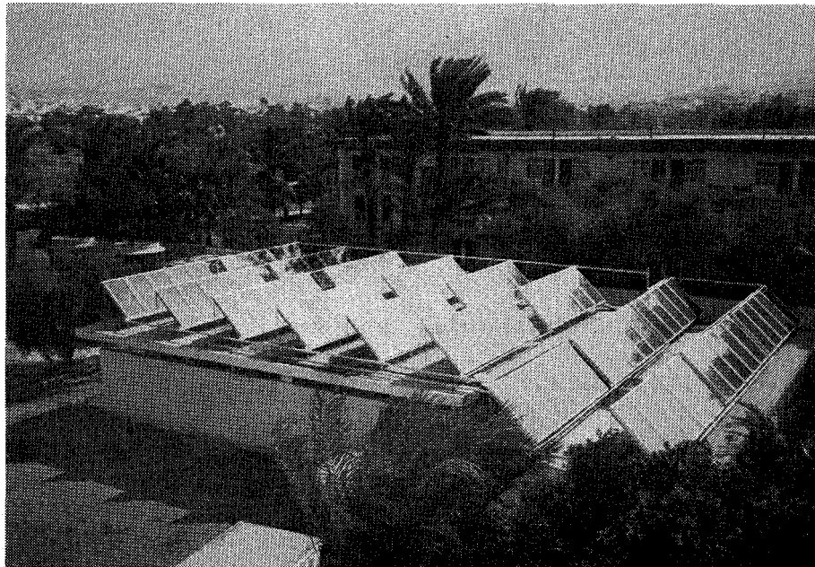
Fig (3.4): A general view of the collector array.
