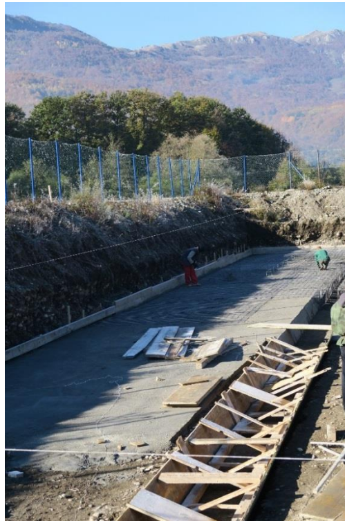
Figure 37: Formwork for the drainage trench placed in the middle of each bed
