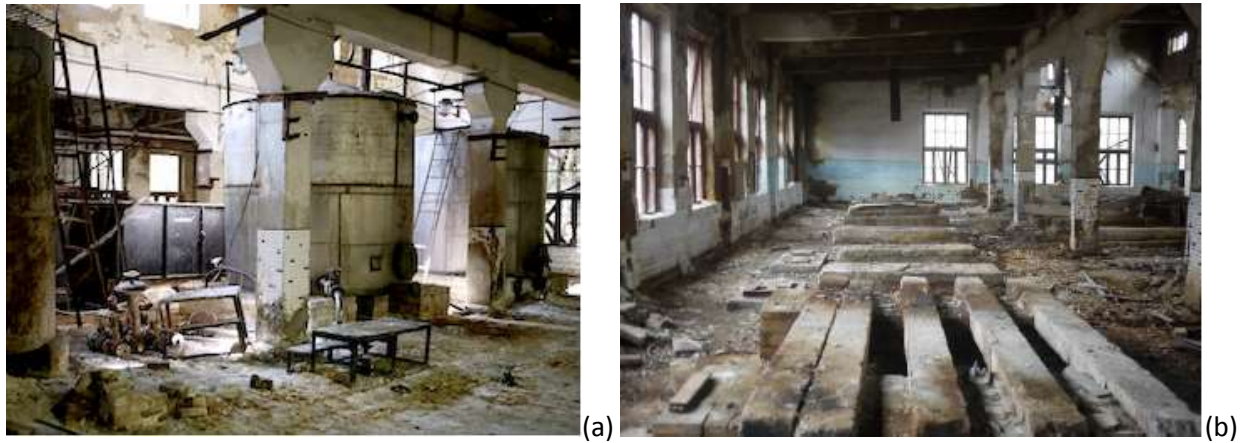
Figure 2: (a) Interior of building 7a before dismantling and removal the TNT production equipment, and (b) after removal of the TNT production equipment
