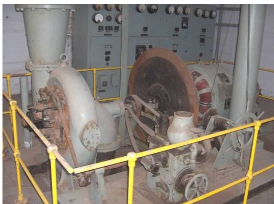
Figure 5 Interior of the decommissioned Hartbeespoort plant in South Africa
