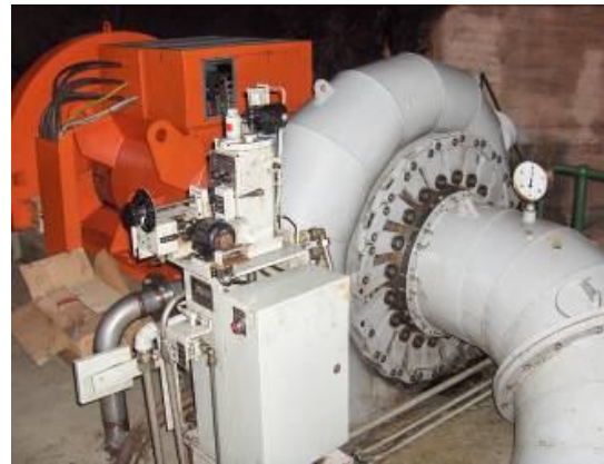
Figure 3 Powerhouse of the Mantsony'ane hydropower plant in Lesotho
