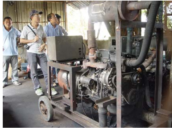
Figure 15: Sim Chanrith generator set
