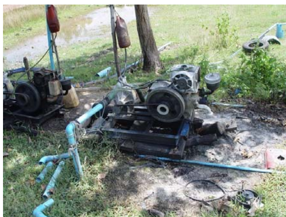
Figure 27: Diesel fuelled water pump
