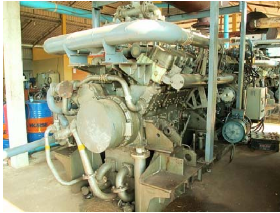
Figure 19: Gas generator 1.25 MVA
