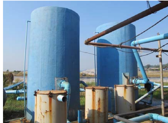
Figure 18: Gas treatment system
