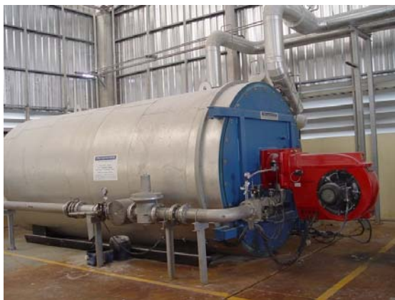
Figure 11: BAI thermal oil heater
