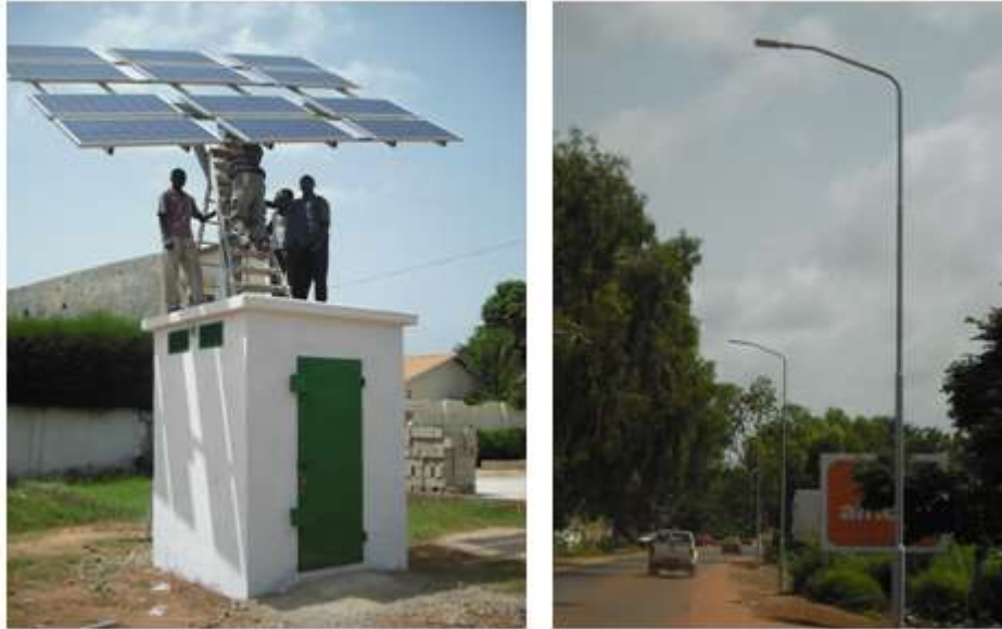
Figure 4 : Solar power Streetlights along the Bakoteh road
