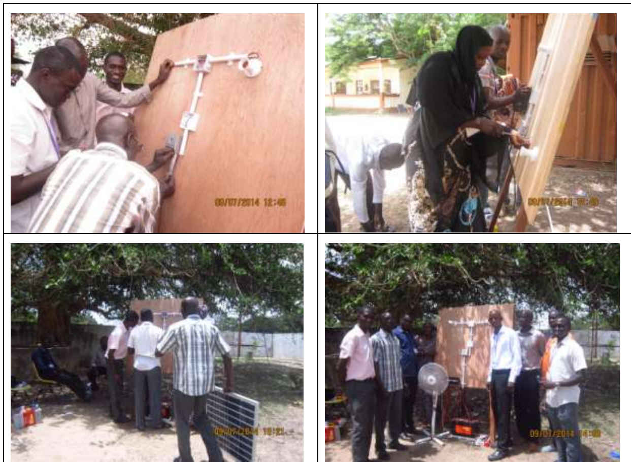
Figure 5 :Participants installing a solar PV system with connected loads during the practicals
