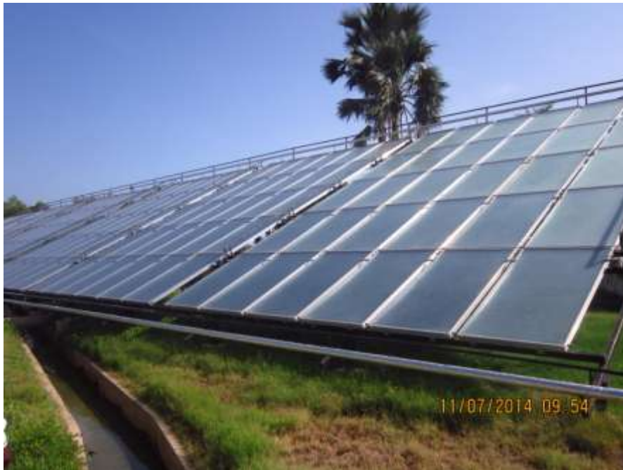
Figure 6 : large solar water heating system at Senegambia Hotel
