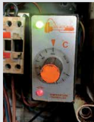
The temperature controller used for this case study. Both this item and the energy meter also used in the case study cost R 1100.
