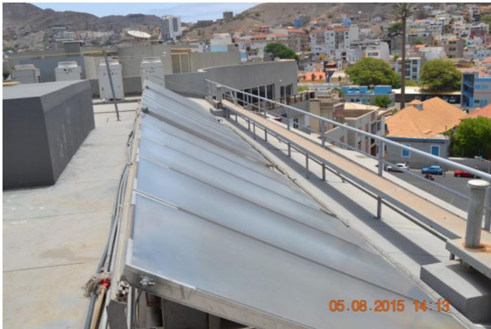
Figure 28: CPC AO SOL collector field mounted in a metal structure on the terrace of Dom Paco Hotel
