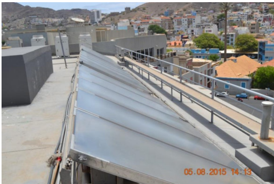
Figure 7: DOM PACO Hotel (44 rooms with capacity for 80 guests) – 15 collectors from CPC AO SOL with individual area of 2.51 m 2 , or 37.65 m 2 equivalent to 26.4 kW. The system supplies hot water to rooms, laundry and kitchen services.
