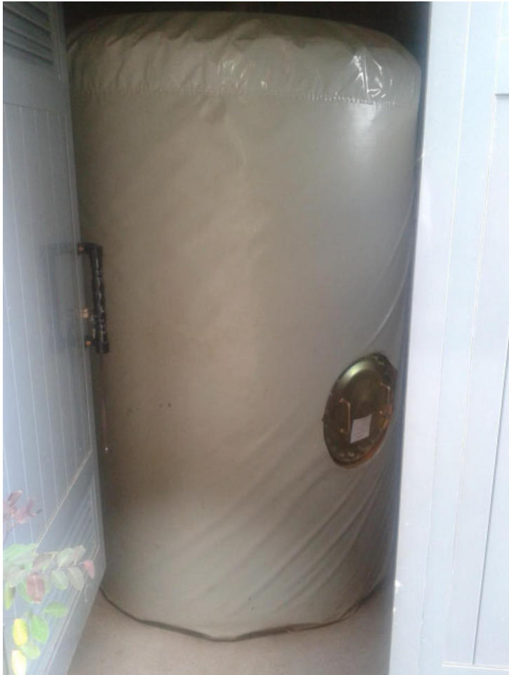
Figure 15: Well insulated storage tank PESTANA TROPICO HOTEL
