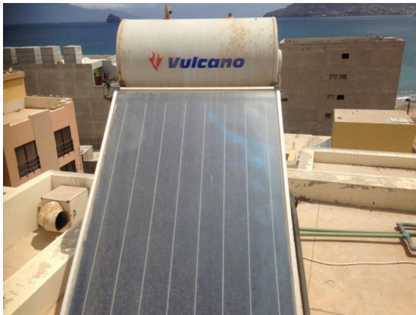
Figure 3: 150 liters thermo syphon indirect type solar collector mounted in small hotel
