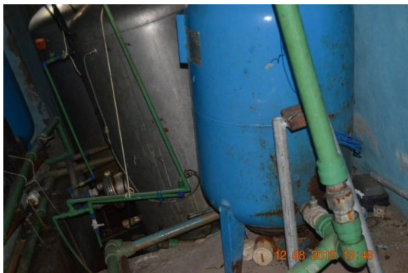
Figure 10: MINDEL Hotel – storage tanks and distribution piping uninsulated
