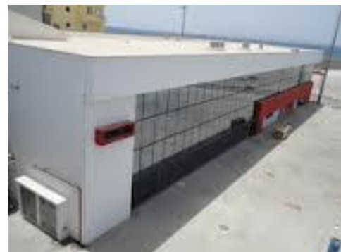
Figure 24: Passenger Maritime Station of Porto Novo, Santo Antão – south and west façade glassed. The installed AC units revealed inadequate during operation. AC Condensers placed in the searing heat of the roof.
