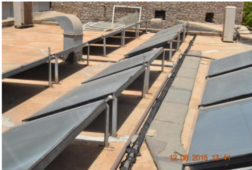
Figure 9: MINDEL Hotel, poorly insulated copper piping carrying hot water to storage tank
