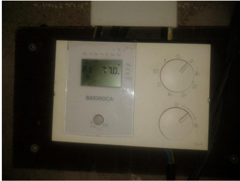
Figure 16: Temperature controller PESTANA TROPICO HOTEL
