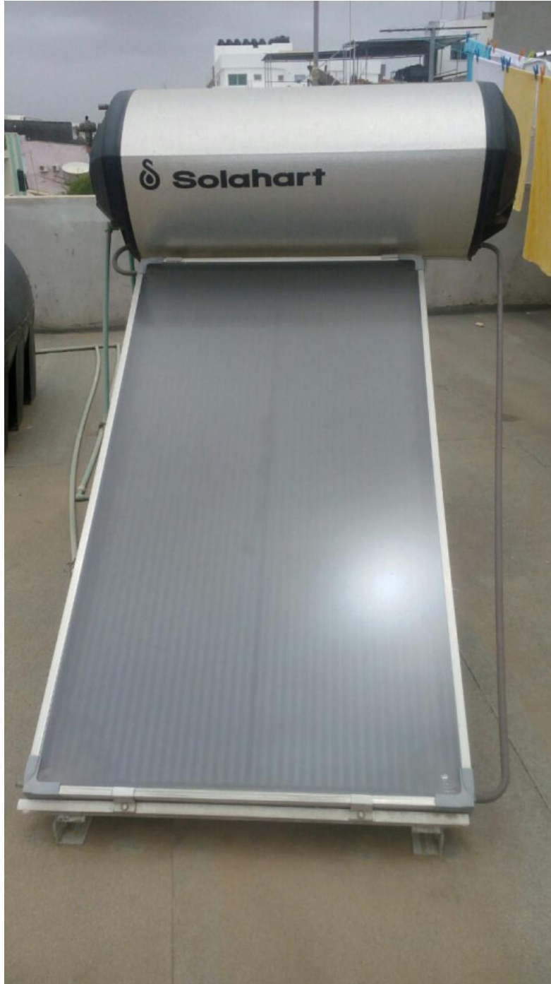
Figure 11: Rotterdam Hotel in Praia – 1 x 180 liter solar SOLARHART collector
