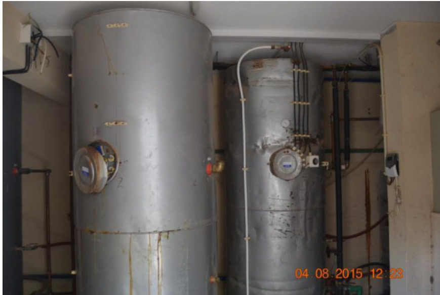
Figure 6: 3 x 1,000 liters storage tanks for above system (FOYA BRANCA Hotel, S. Vicente).
