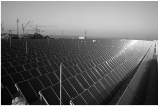
PICTURE 2. OVERVIEW OF THE 36.305 \text{M}^2 ROOF MOUNTED SOLAR THERMAL COLLECTOR FIELD ON TOP OF A HUGE WAREHOUSE (PICTURE SOURCE: MILLENNIUM ENERGY INDUSTRIES).
