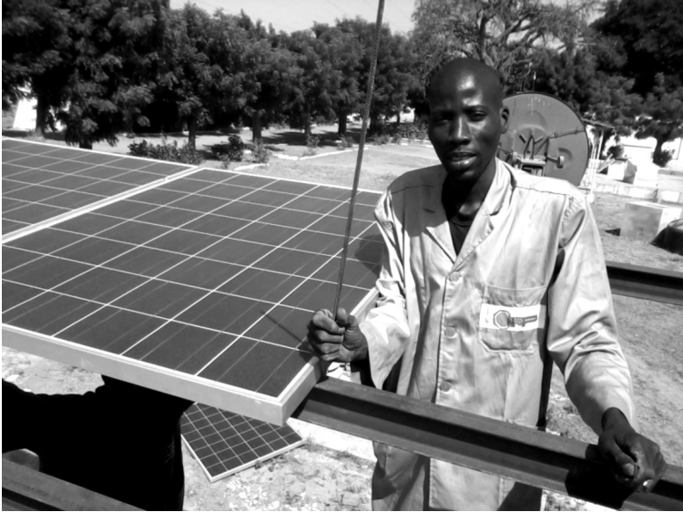
PICTURE 10. TECHNICIAN OF THE LOCAL INSTALLER COMPANY WORKING ON THE 3 kWp INSTALLATION IN CERER. NOVEMBER 2012.
