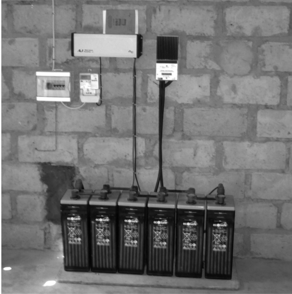
PICTURE 5. INTERIOR EQUIPMENT OF THE TECHNICAL ROOM. FORDOU.
