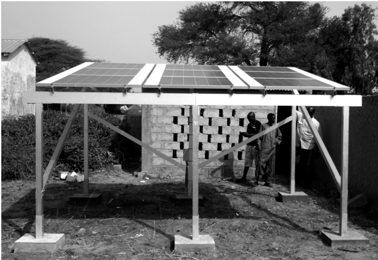
PICTURE 4. PV INSTALLATION AND TECHNICAL ROOM. FORDOU.
