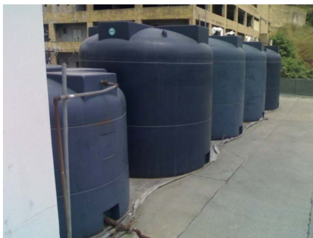
Uncontrolled water supply at the roof of a food industry in Mount Lebanon
