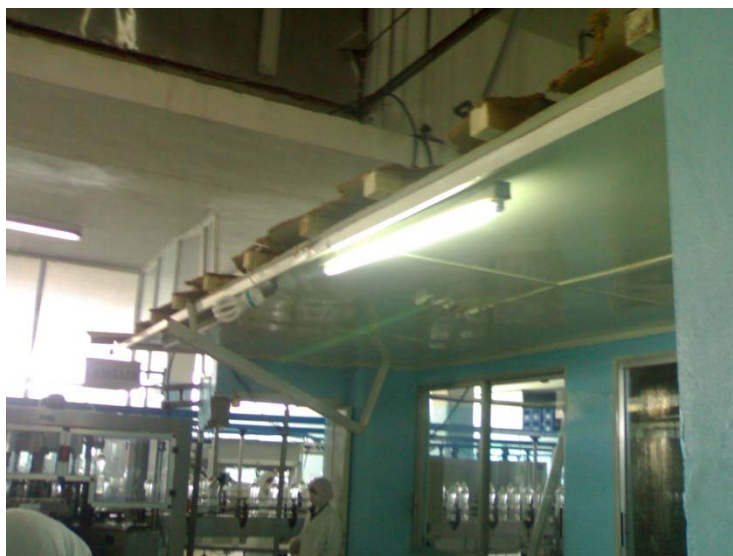
Unnecessary suspended damaged sealing and fittings just besides filling operation of food product
