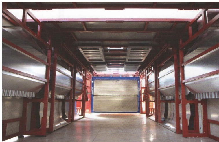
Figure 57. Toggle dryer, of the Cell Rotaring Conditioning (CRC) System, inside view
