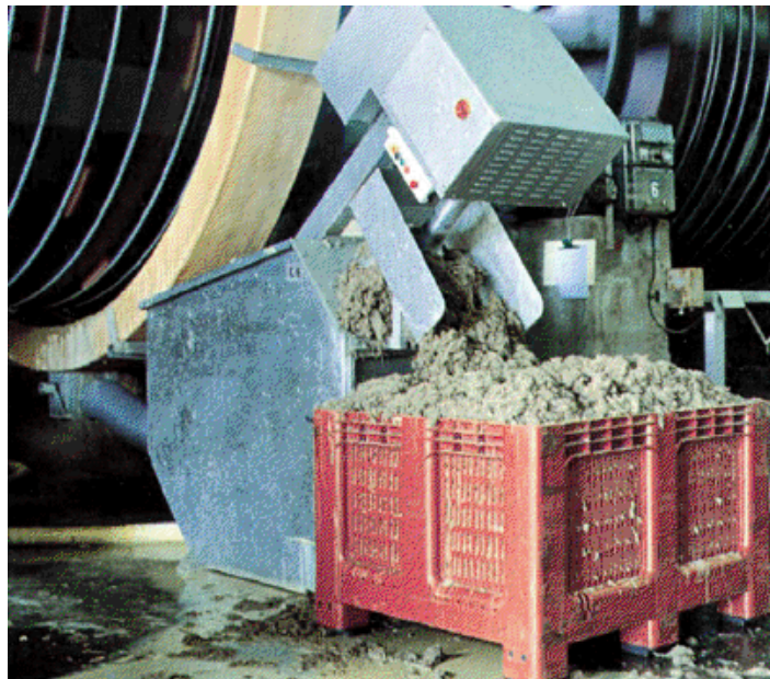
Figure 28. Screw type screen with compactor and container
