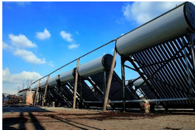
Figure 77. Solar collectors installed in a tannery under UNIDO project in Bangladesh
