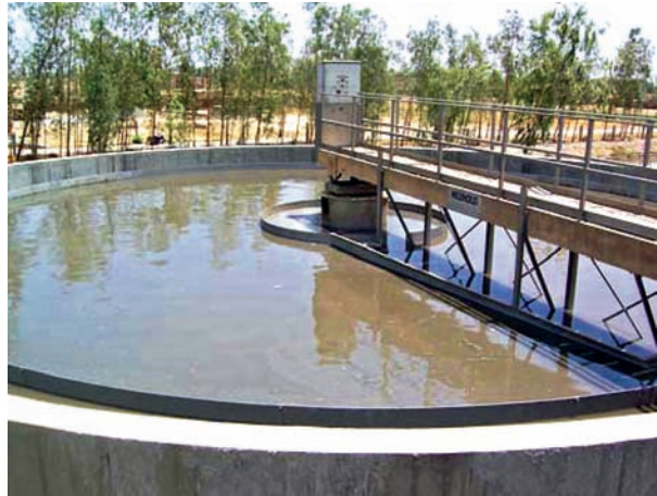
Photo 4. Sedimentation tank in operation
