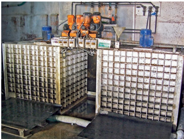
Photo 1. Coagulant/flocculant dosing station
