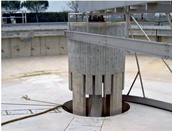
Photo 3. Sedimentation tank (empty)
