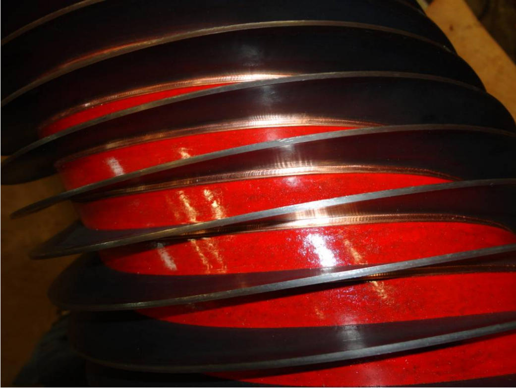
Figure43 Caulking in correct position. Note that hammer has been hitting the caulk only with an even result
