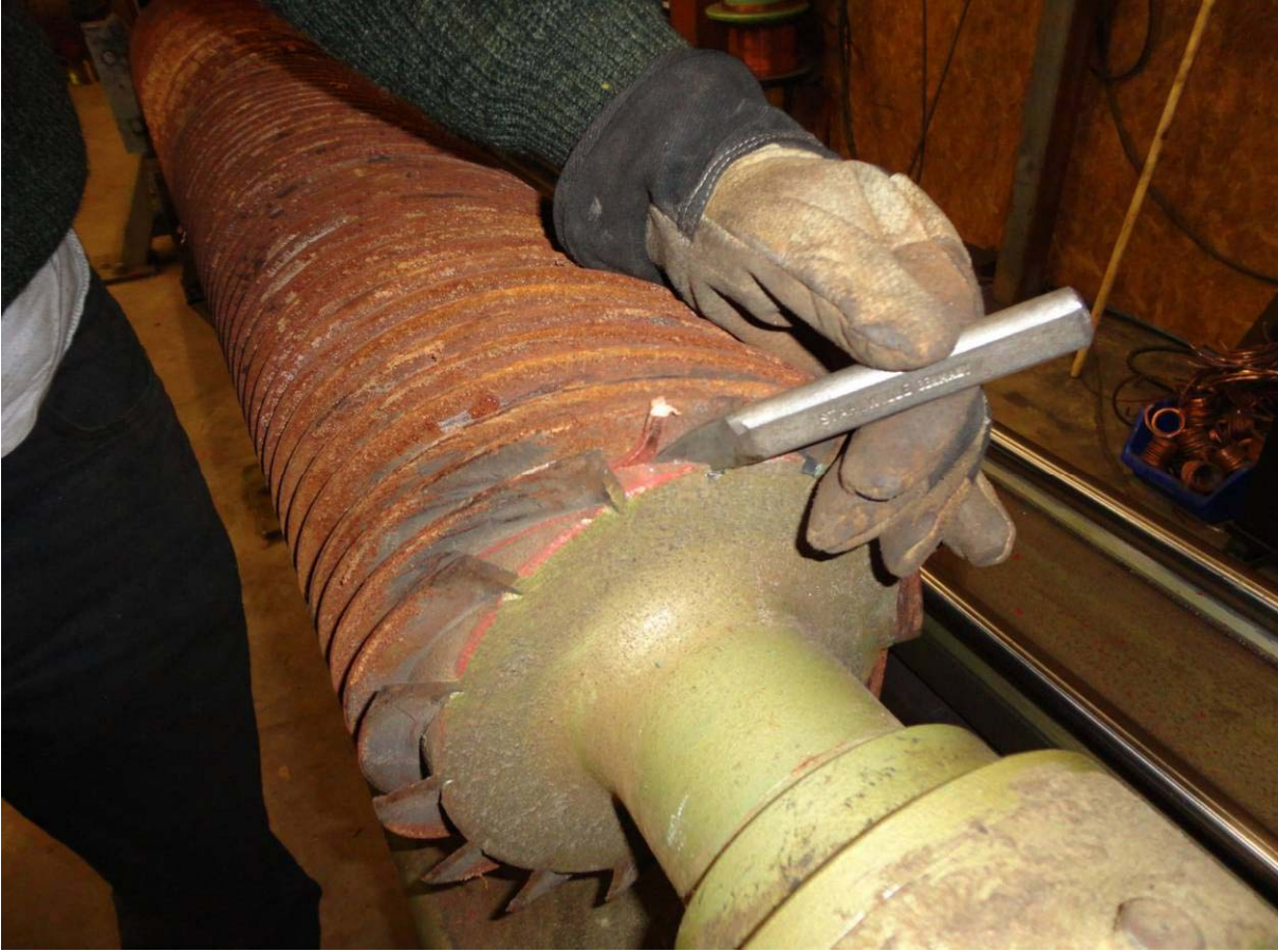
Figure 8 Lift enough of the caulking that you can grab it with pliers
