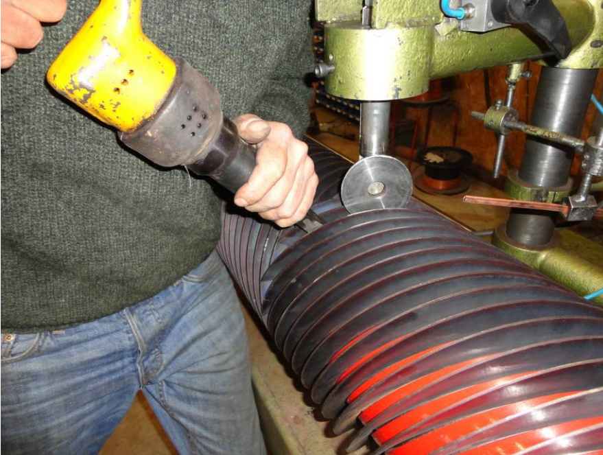
Figure 38 Fastening of blades with pneumatic hammer. Note steel wheel on the blade top, holding the blade in the bottom of the groove
