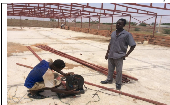
One Welding Group from the old beneficiaries are taking big contracts, building a Skelton of a Chicken Farm
